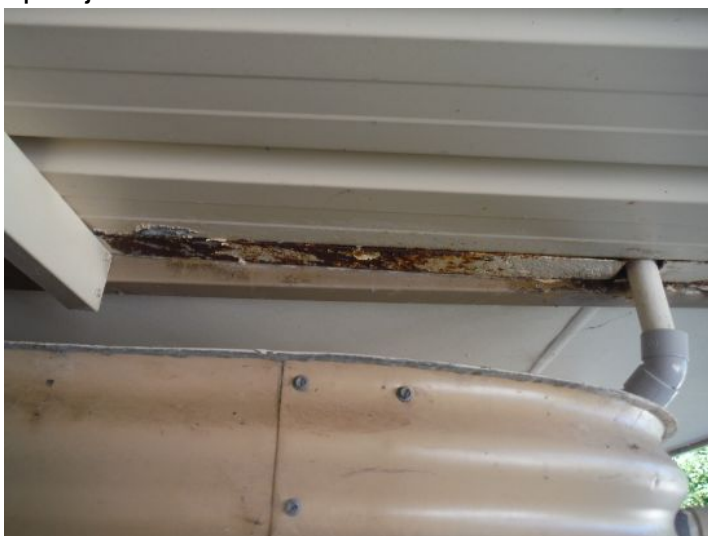
Some corrosion noted at the patio outside the laundry. Recommend maintenance.
