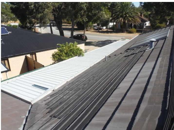
Old system still present.
