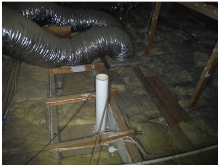
Kitchen extractor pipe.
