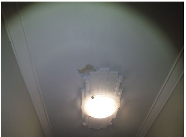
Stain noted at the hallway light
