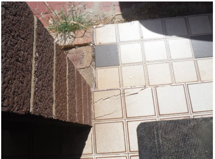
Crack at front porch steps noted.
