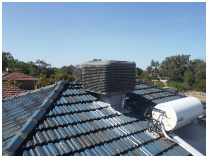
Monitor the AC unit when in use. Stains noted. This may be leaking.
