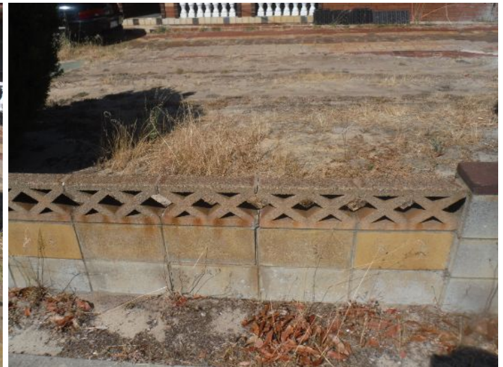
Small vertical crack noted.
