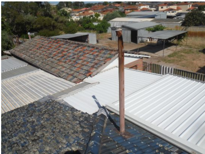
Noted the vent pipe has corroded. Recommend maintenace
