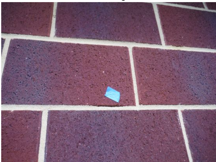
Mortar needs touching up on the East wall.
