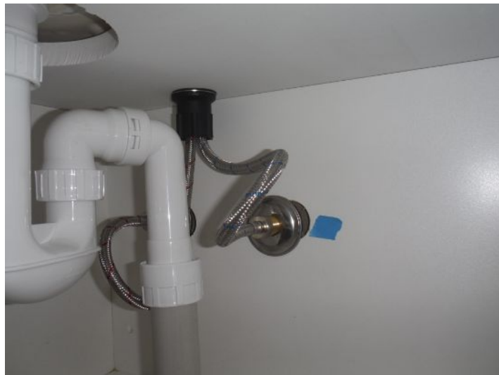
Noted hole at the main bathroom sink back. This needs covering.
