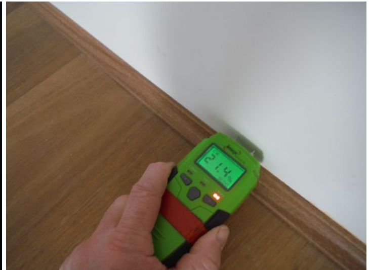
The lounge wall has moisture present at low level from the past ensuite sink leak. Monitor the flooring
