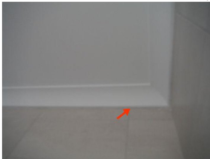
Some shrinkage cracking at the bathroom ceilings to gap fill.
