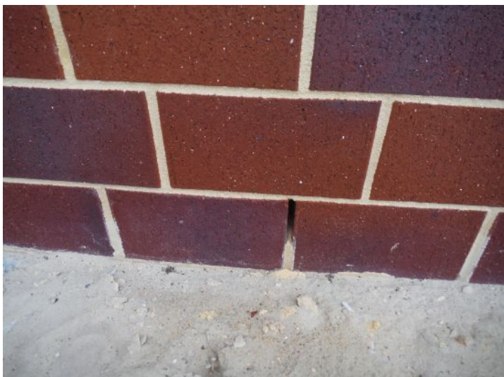
Some weep hole vents need adjustment or installing.
