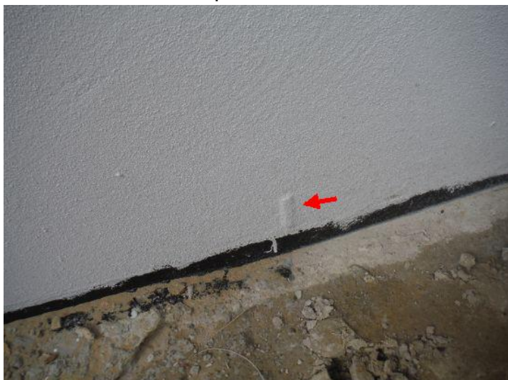
Noted the weep holes need uncovering at the front render.
