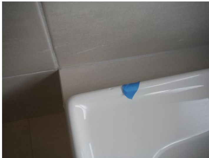
Small chip on the bath needs repair.
