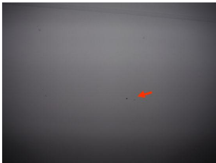
Screw hole to fill in the garage ceiling.
