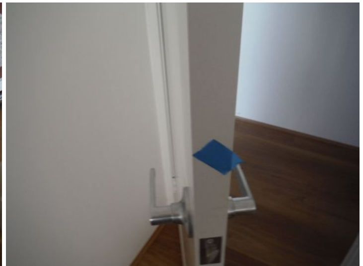
A number of doors have rough edges and need sanding and repainting.
