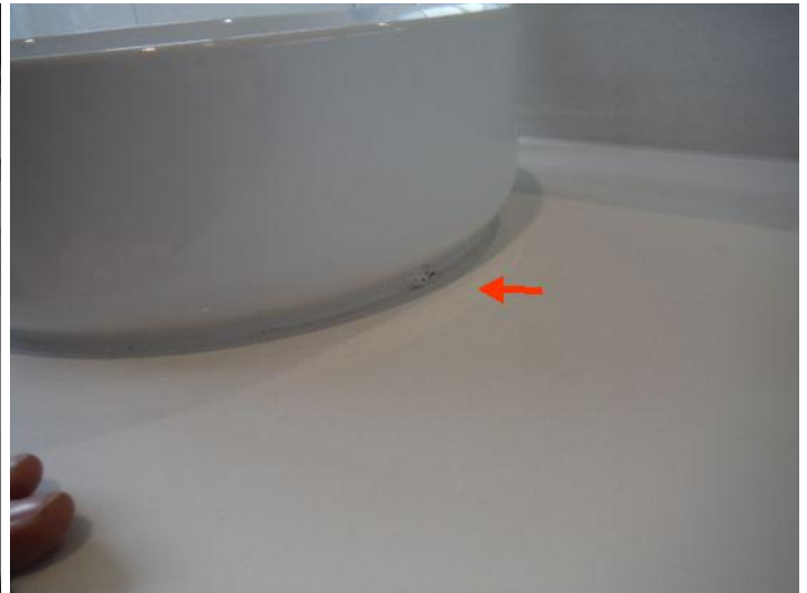
The silicone at the main bathroom sink needs repair.
