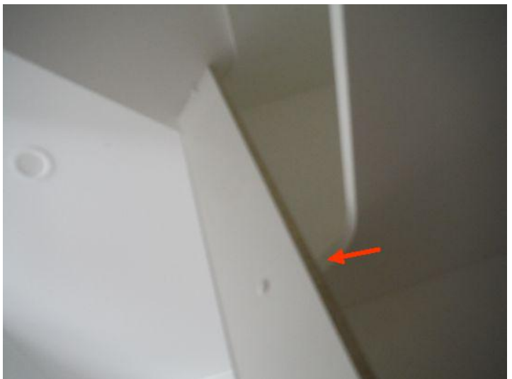
The pantry door timber has no edge trim fitted.
