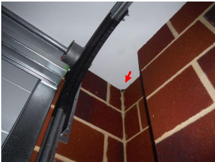
Small hole to fill at the front of the garage ceiling.
