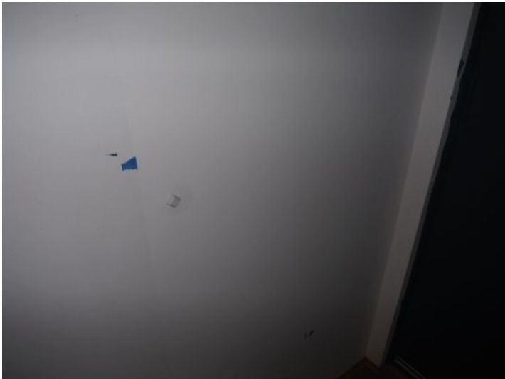
Paint marks at the front door wall to remove.
