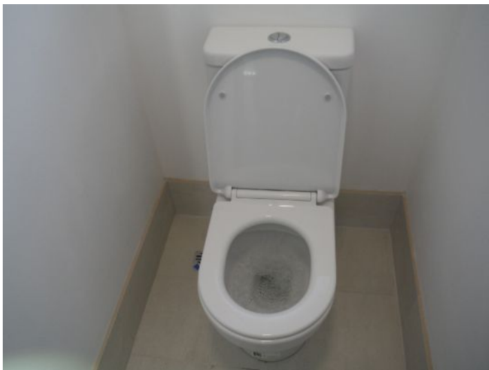
The toilets are slow to drain and need checking by the plumber.
