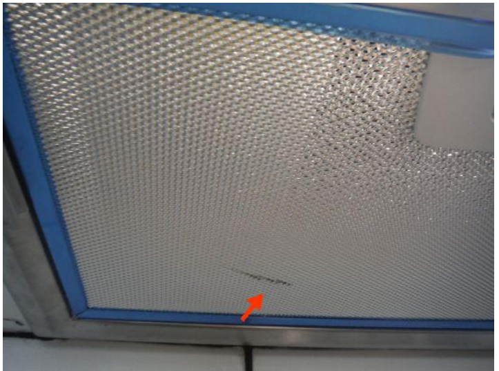
Mark / scratch on the vent mesh grill.
