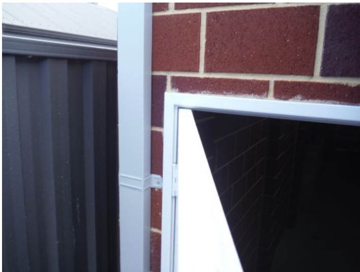
The top of the garage access door needs recoating
