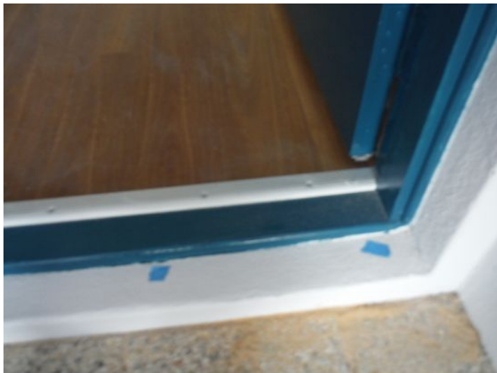
The paint needs touching up externally on the frame.
