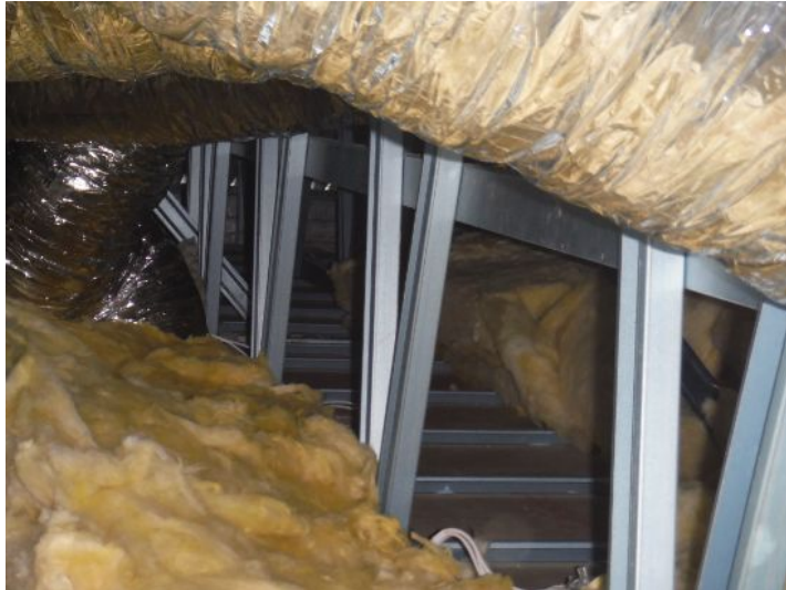
The insulation has been disturbed in areas and needs replacing.
