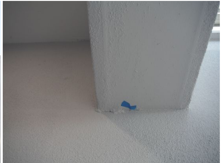
Some excess render and paint on the underside of the porch lintel need cleaning up.
