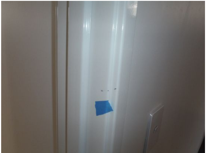
Some door frames need the paint touching up.
