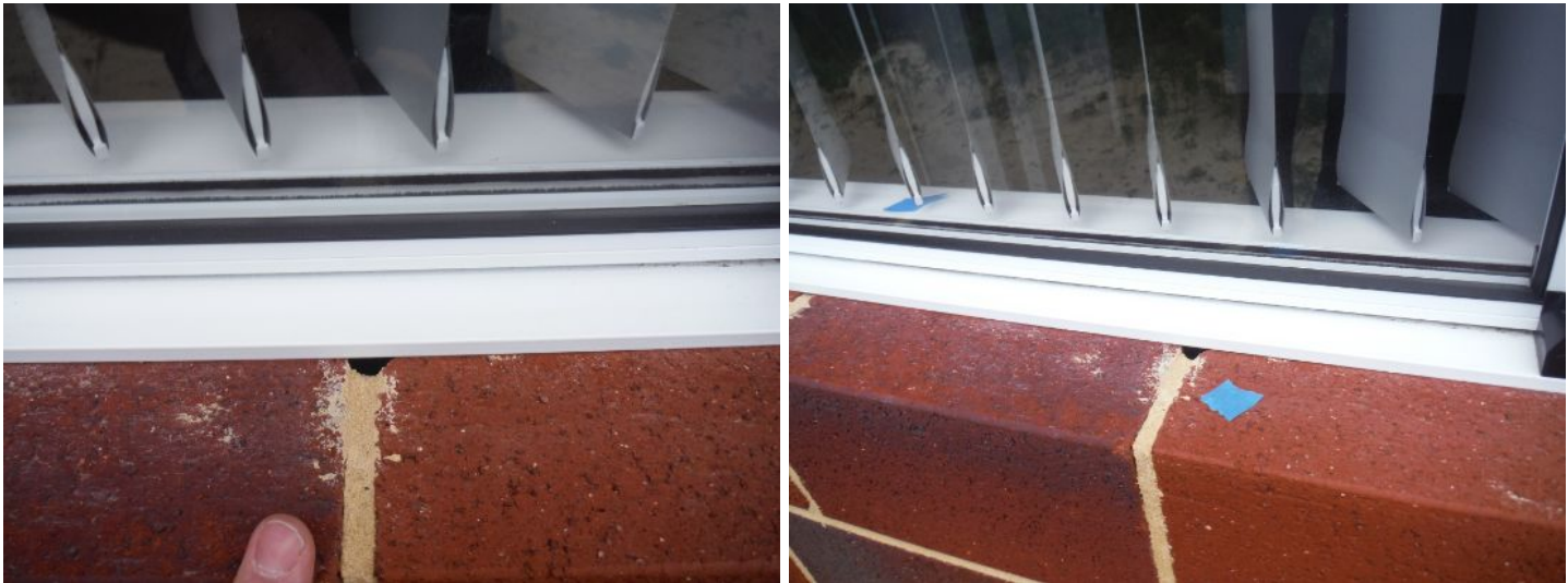
Some mortar on the window sills needs touching up.
