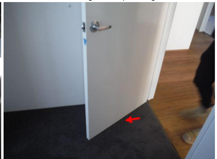
One rear bedroom door needs shortening as its rubbing the carpet.
