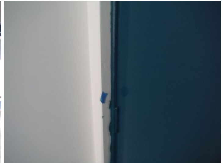
The paint over runs need cleaning up / repainting at the front door.
