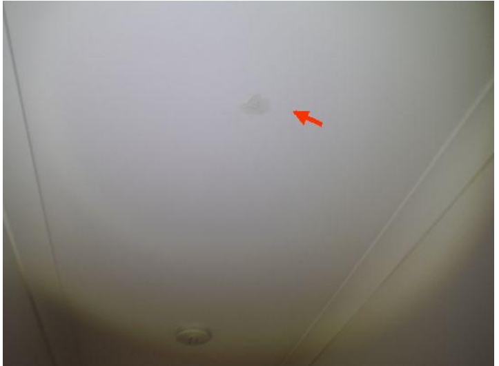
The entrance hall ceiling needs this patch sanded and painted.
