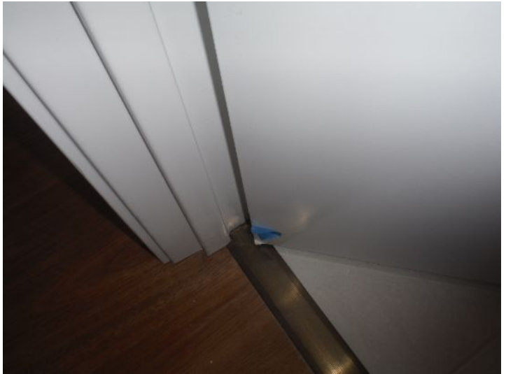
Noted the base of the laundry door needs trimming up.
