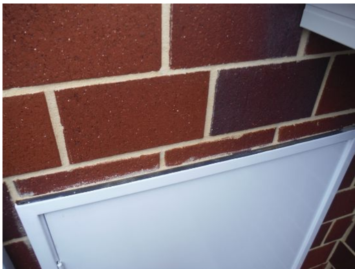
The garage access door head needs painting.
