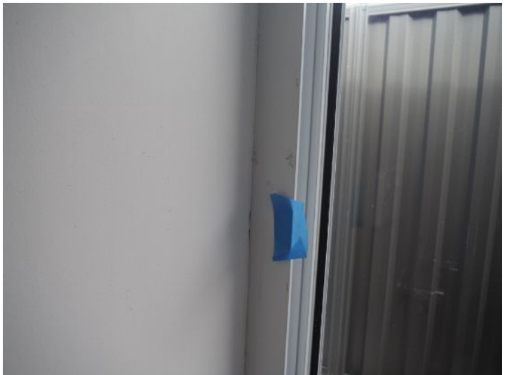
Some marks on the laundry door frame need cleaning off
