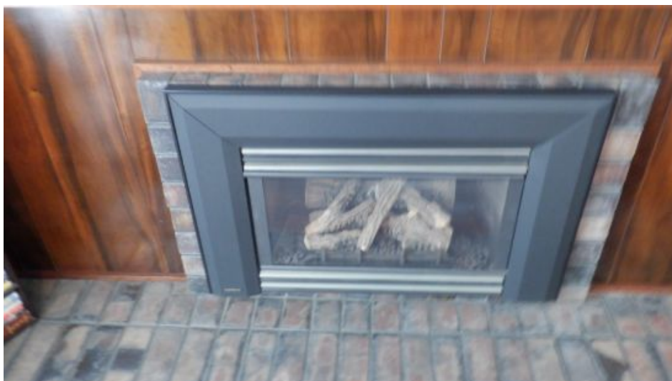
Noted gas fire, not tested in our inspection
