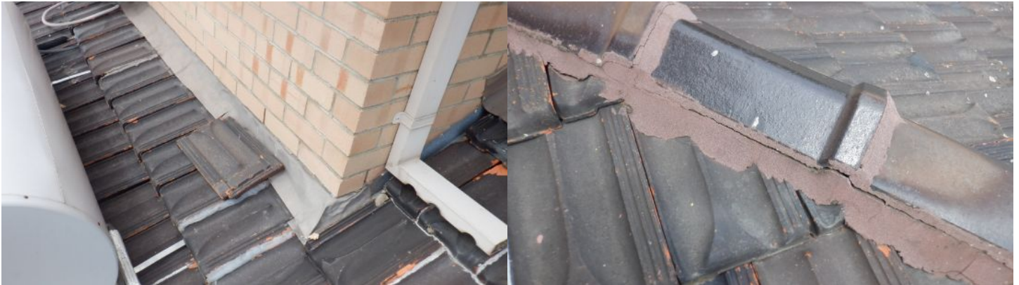
Silicone has been applied to the tile joints below this downpipe area.
