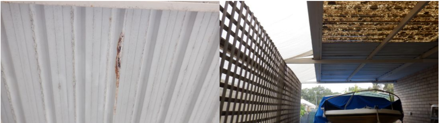
Noted some corrosion below the roof sheets, maintenance
