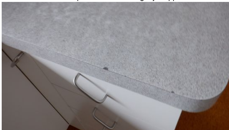
Small chips and wear noted, maintenance
