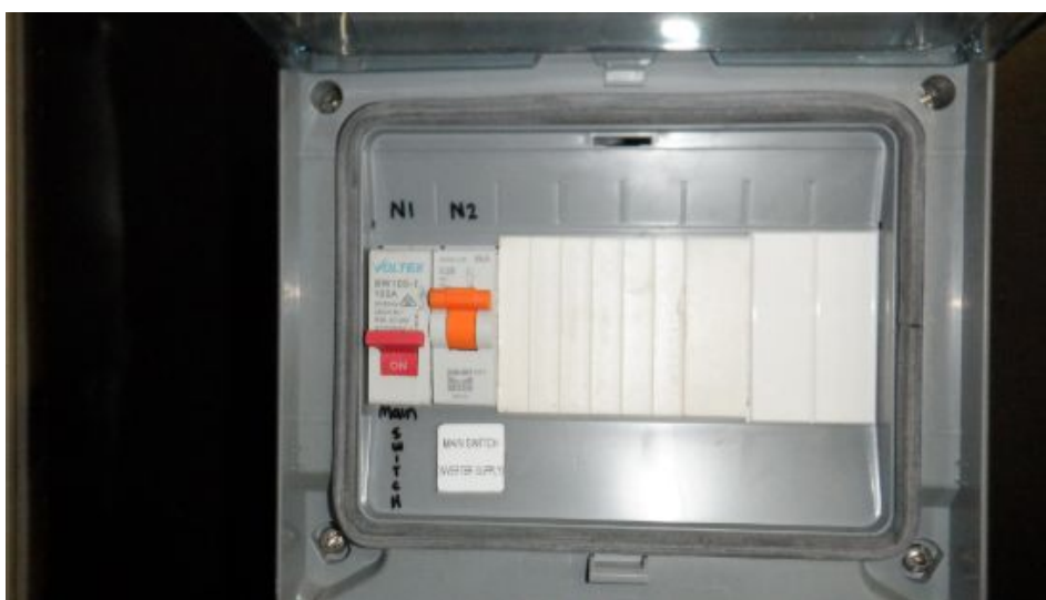
Shed sub panel
