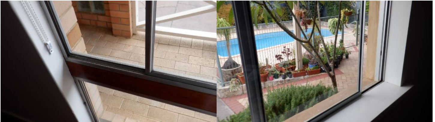
Some fly screens were not installed
